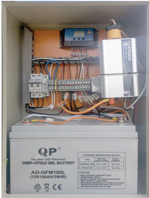
Fig. 5. Photovoltaic system test prototype.
