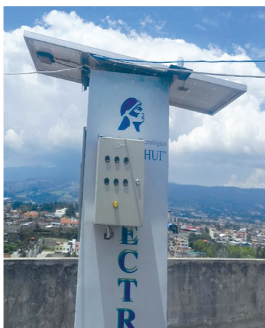
Fig. 3. Photovoltaic system test prototype
