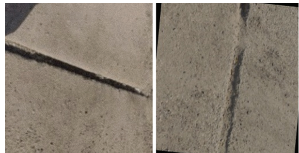
Fig. 30. cracks from illegal drilling from Iraqi streets
