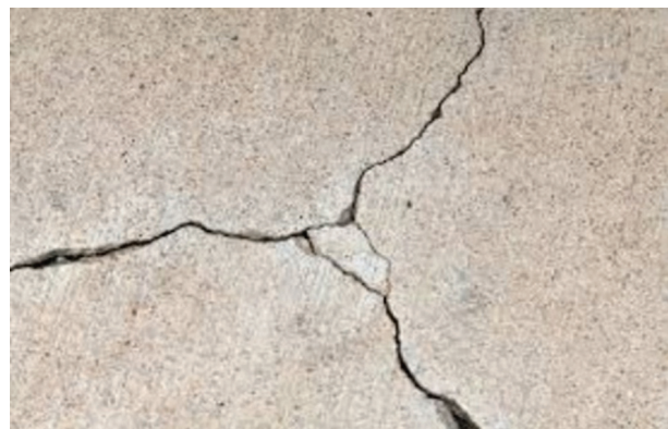
Fig. 27. Crack in concrete surface
