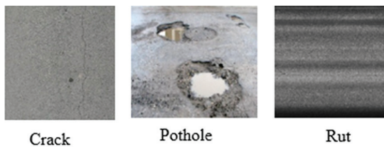
Fig. 10. Three types of asphalt distress under the study
